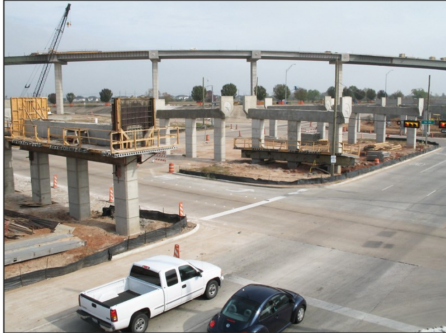
West Park Tollway
